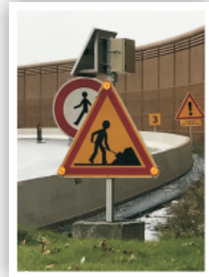
alimentation solaire (sur support)
